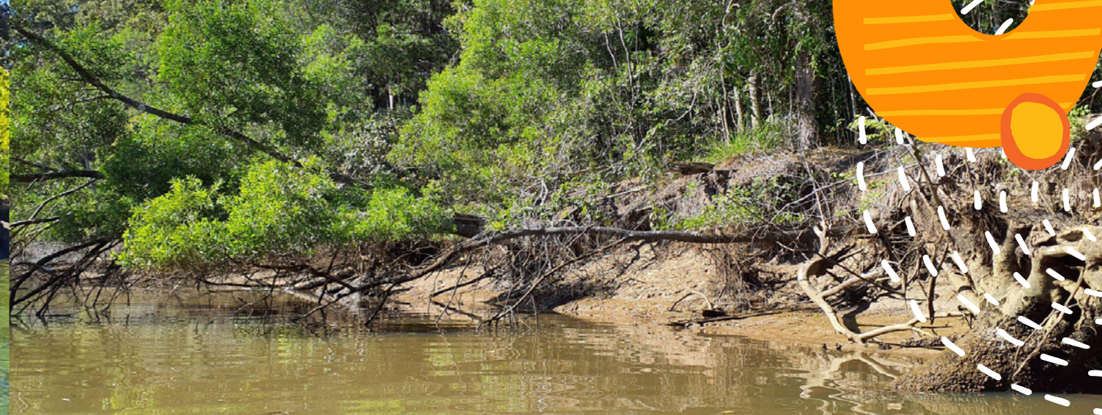
Figure 9. Bank collapse and fallen trees along a stretch of the Brunswick River.
