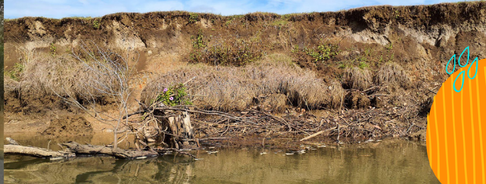
Figure 12. When riparian habitat is entirely cleared - it can have a disastrous impact on riverbank stability and erosion, especially when cattle have unrestricted access to the water.
