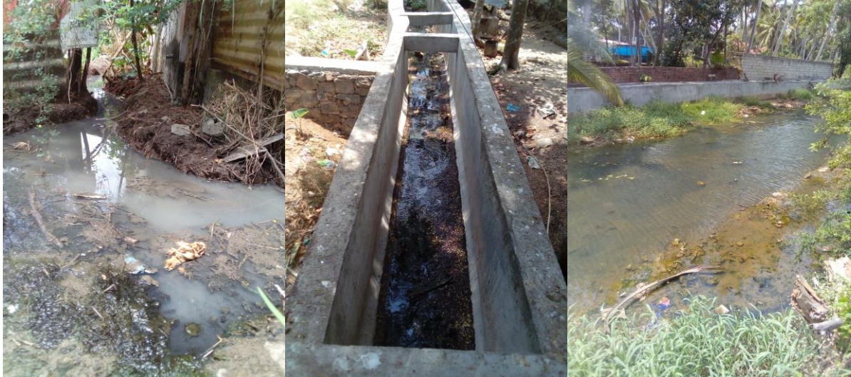
Figure 10: From left to right: Sewage accumulation area, sewage infrastructure, channeled part of the river
